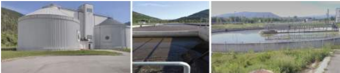
Fig. 2 Methane tanks, biobased area with aerobic and anaerobic digestion zone, secondary settler
